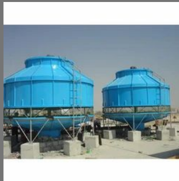
FRP Cooling Tower
