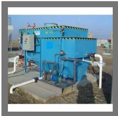
Effluent Treatment Plant
