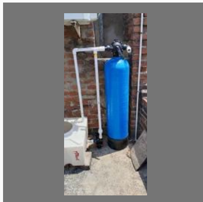
ETP PLANT FOR PATHOLOGY
