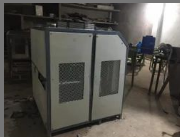
Industrial Water Chiller
