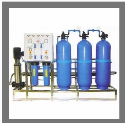
Industrial Ro Plant
